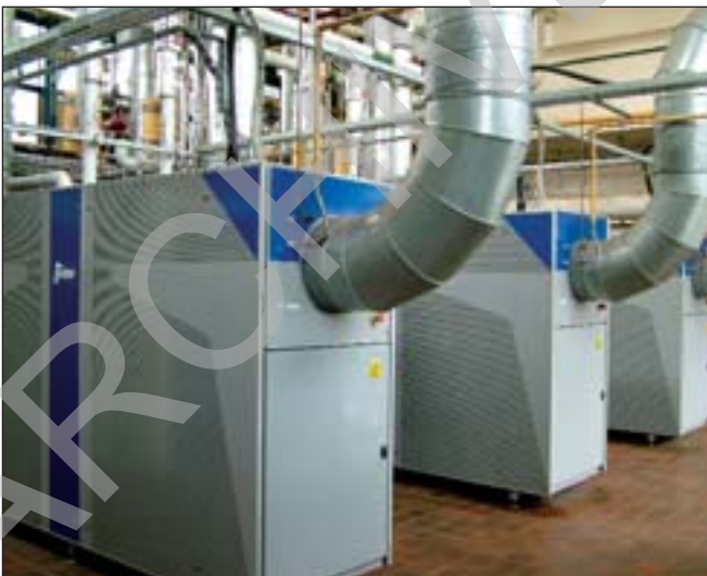
Nevill Hall Hospital, Gwent Healthcare Trust. Micro-turbine combined heat and power plant. Six micro-turbines – each rated at 100 kW electrical and 150 kW thermal output. The units can be sequenced much like a modular boiler installation. Electricity is used to offset import requirements and the heat output services heating and hot water demands in the winter and cooling in the summer
