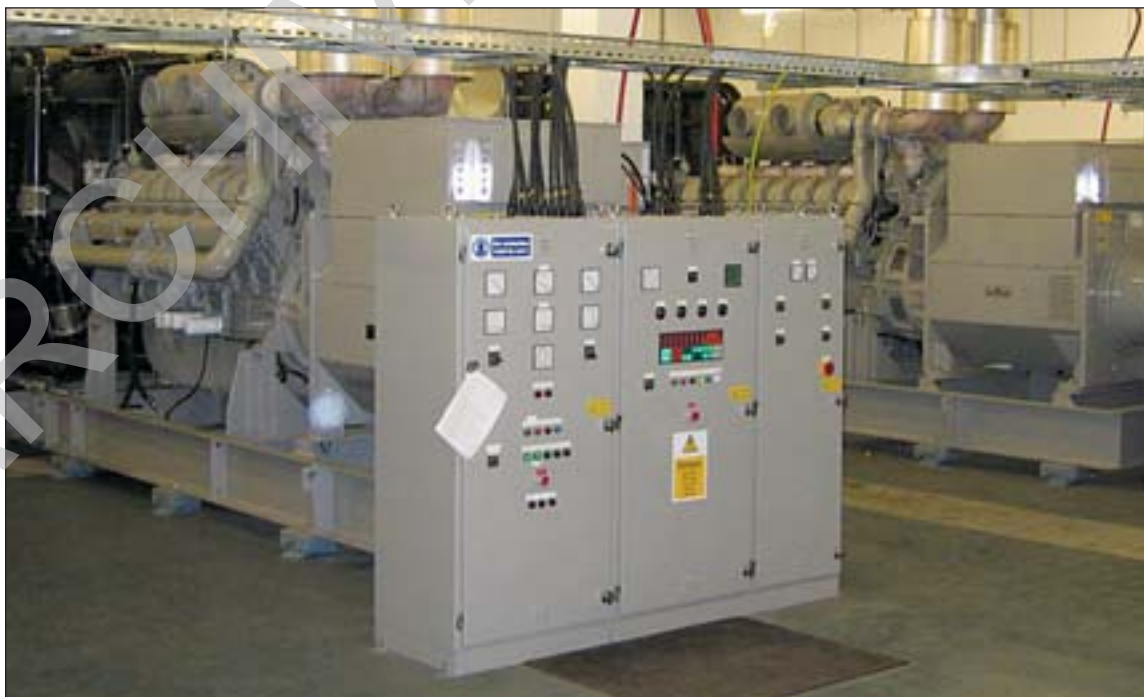
Princess Royal Hospital, Bromley. A view of the standby electricity generator plantroom showing good access space for maintenance etc
