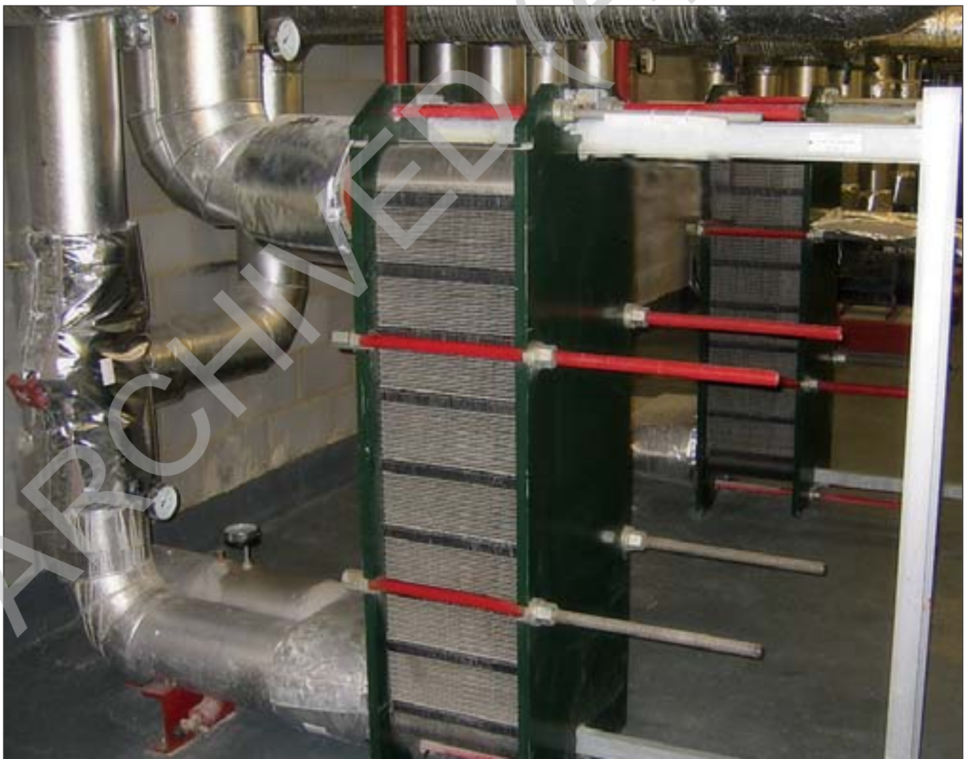
Princess Royal Hospital, Bromley. A view of plate heat exchangers in a plantroom at the Princess Royal Hospital
