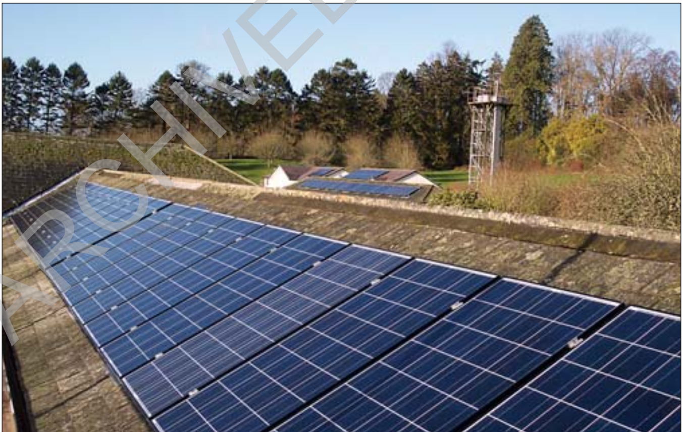
Photovoltaic installation at Bronllys Hospital, Powys. Courtesy of Powys Local Health Board and Welsh Health Estates
