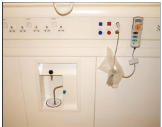
Each bedhead should have outlets for medical gases and vacuum, and (where required) be plumbed for dialysis-standard water, and have drainage outlet points
